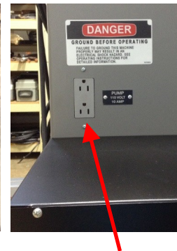
120VAC receptacle for pump
